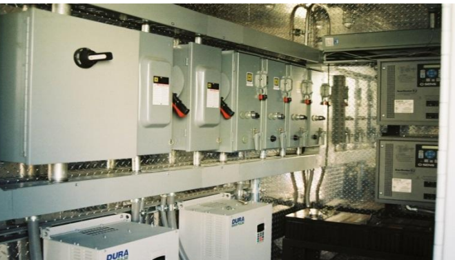
On-Site Utility Grade Power
