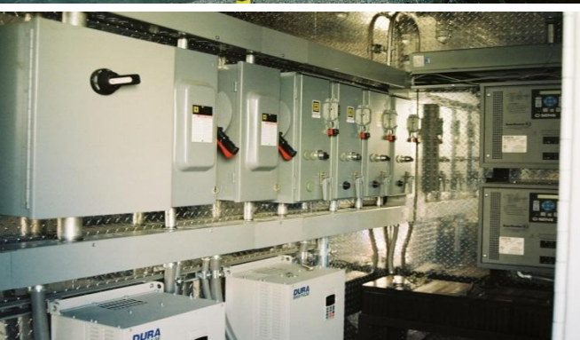
On-Site Utility Grade Power
