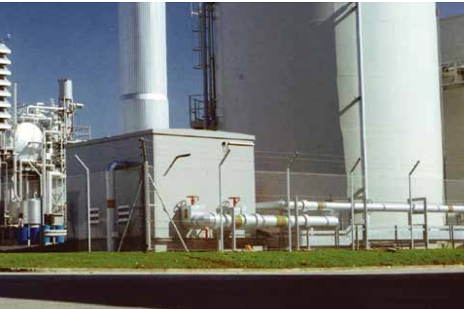
UK power plant utilizes the efficiency and flexibility of the Industrial Trent 60
