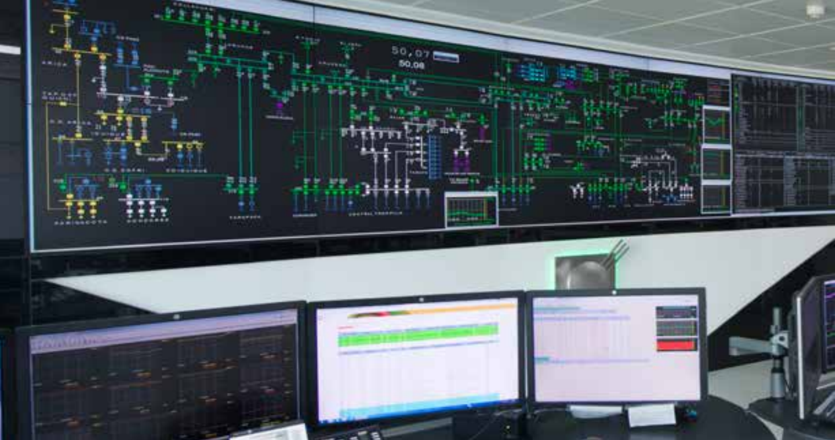
Control Room, CDEC-SING
