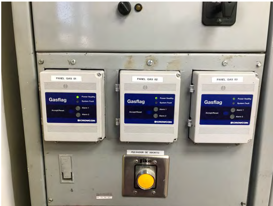
GAS DETECTOR PANEL
